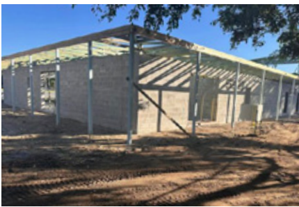
Pictured: Construction of dressing sheds and change rooms at the Burleigh Bears field. Source: Facebook / Cr Nick Marshall OAM Division 12, Gold Coast.
